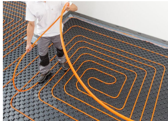
Hot water under-floor heating
